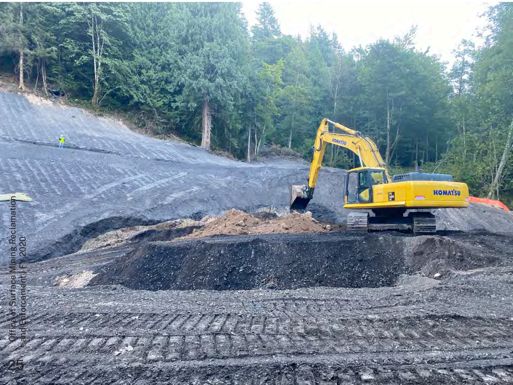
Photo: Heavy equipment at the Navy Mine location working with top soil and spoil grading the reclaimed area.
