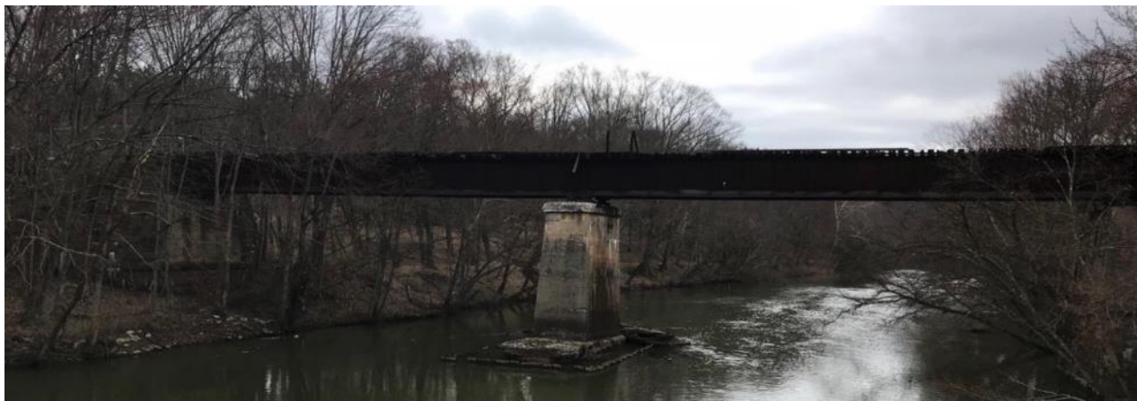
Railroad Bridge to be restored as part of the trail developed with the Porter Floodplain Restoration Project Photo Credit: Pennsylvania Department of Environmental Protection
