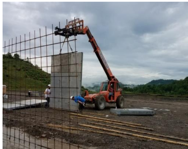
Marion Branch Industrial Park Worksite. Photo Credit: Kentucky Division of Abandoned Mine Lands
