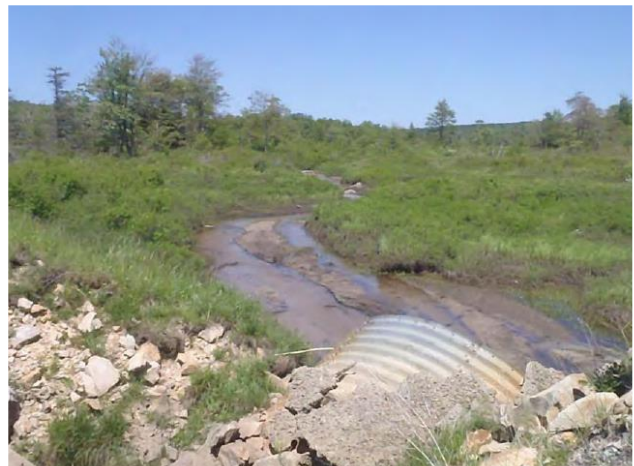
Buffalo Coal Site along Beaver Creek Photo Credit: West Virginia Division of Highways
