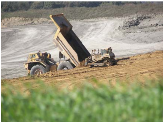
Soil material being replaced over graded spoil as part of the land reclamation process.
