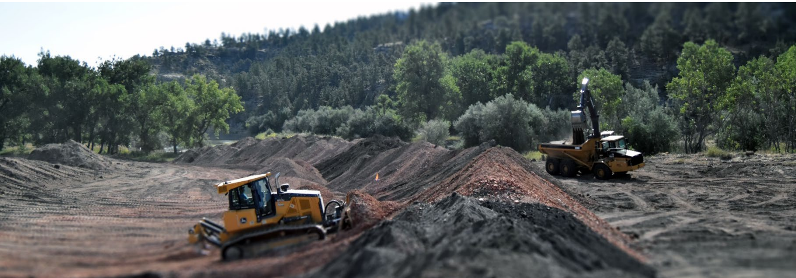
GPS-assisted equipment excavate approximately 47,500 cubic yards of material at the Bair-Collins Mine Reclamation and Floodplain Restoration Project in Roundup, Montana. Photo courtesy of Montana Department of Environmental Quality.
